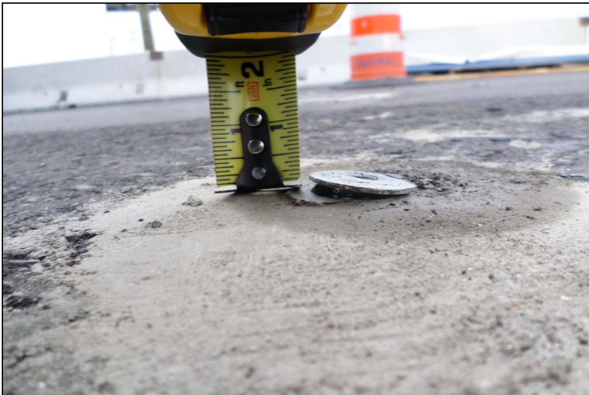
Photo 12 Close-up of 1/8 in. displacement of washer and bolt sleeve assembly at test tie down No. 1.
