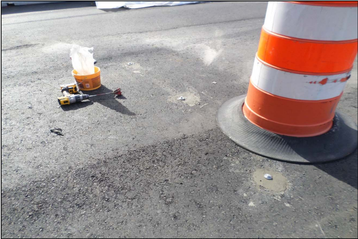
Photo 4 View of three SP12 test anchors installed adjacent to the ICTF Trailer, numbered 3, 2, 1 from left to right.
