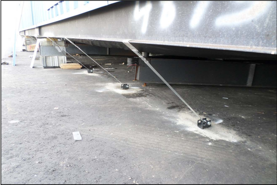
Photo 2 View of typical storm tie downs at the Greenville Yard ICTF Trailer.
