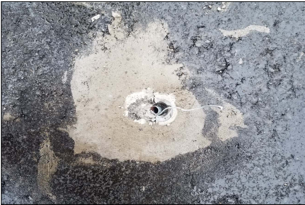
Photo 10 Looking down at broken mounting bolt sleeve at test tie down No. 2.
